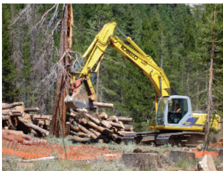
A backhoe stacks logs, some of which will be used in construction of the new stream channel at High Meadow (USFS)
