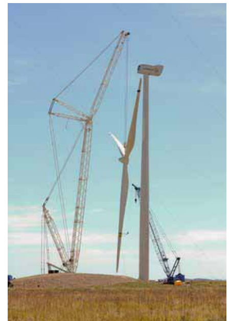
Towers are being lifted as work continues on the 2 MW Gamesa wind turbine that is being installed at the NWTCC. Credit: NREL
