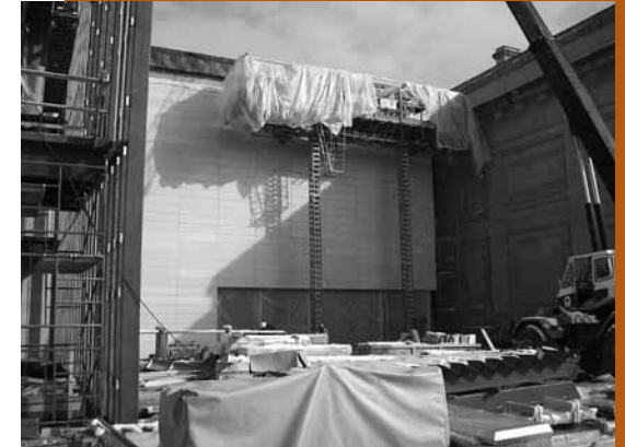
A Davenport Masonry employee fell to his death while working from this scaffolding.
