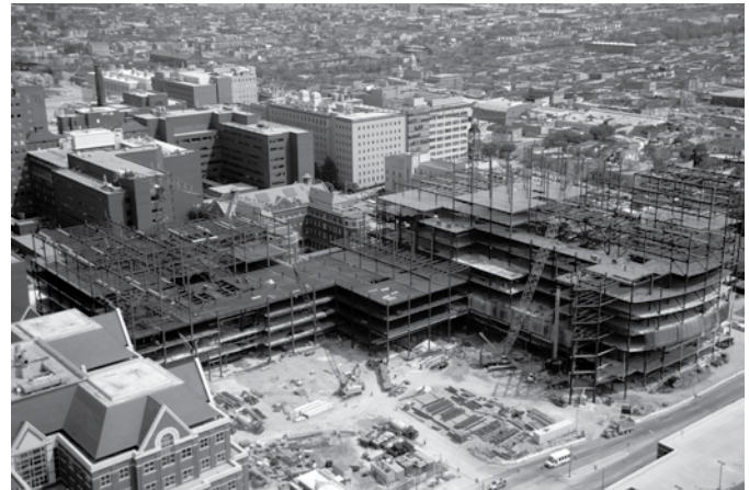
The New Clinical Building is one of the largest commercial construction projects in Maryland.
