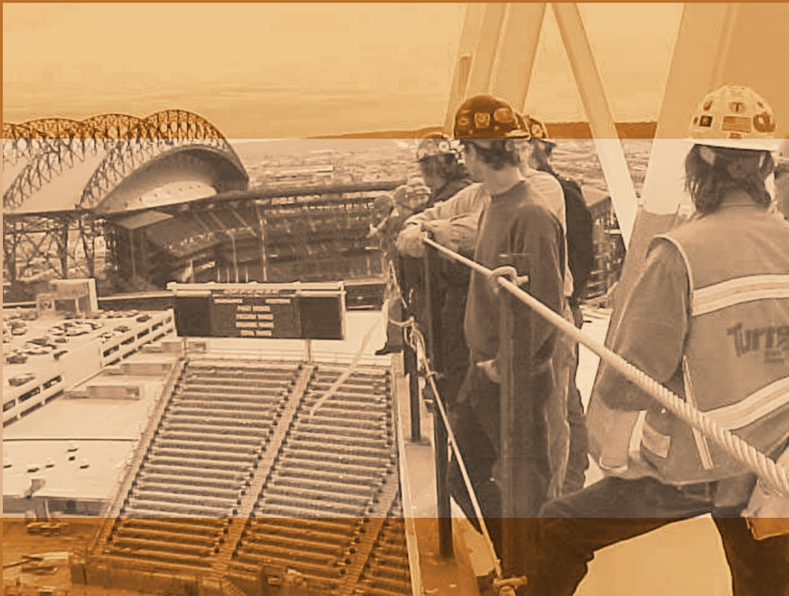
Fall protection — overlooking Safeco Field — Washington
