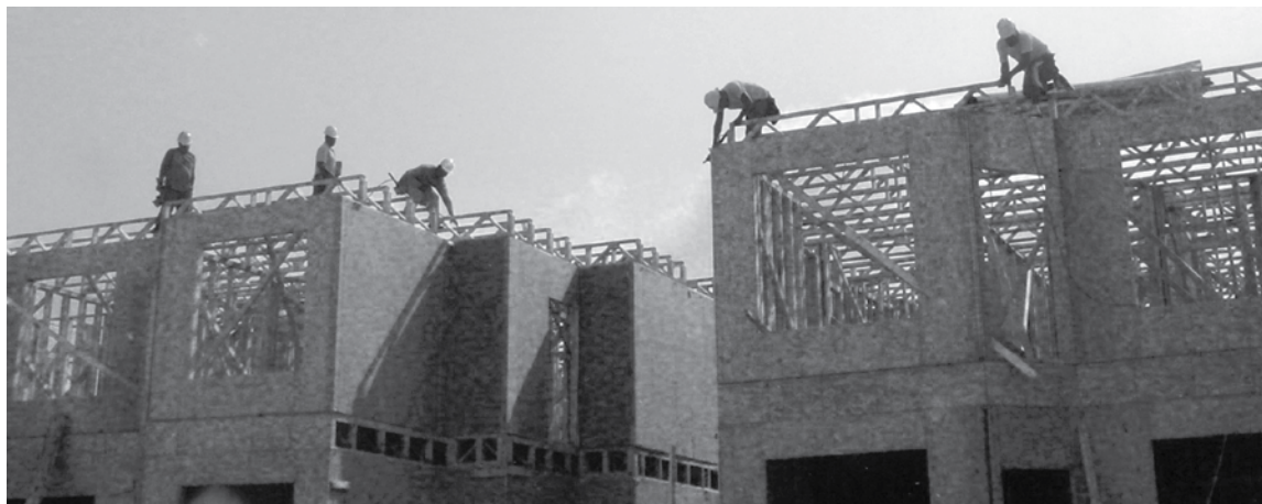
Fall protection is the most serious hazard in residential construction. South Carolina OSHA conducts quarterly construction focus inspections throughout the state.
