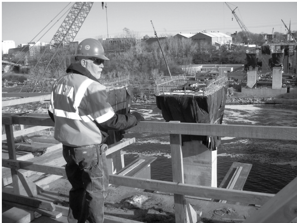
A Minnesota OSHA investigator checks guardrails during a visit to the I-35W bridge rebuild site.
