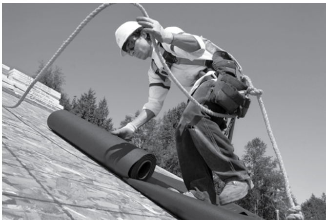
Pedro Vargas uses a harness and rope to make sure he is safe while rolling out tarpaper on the roof of a new Quadrant home in Mount Vernon. Photo by Meryl Schenker, used with permission.
