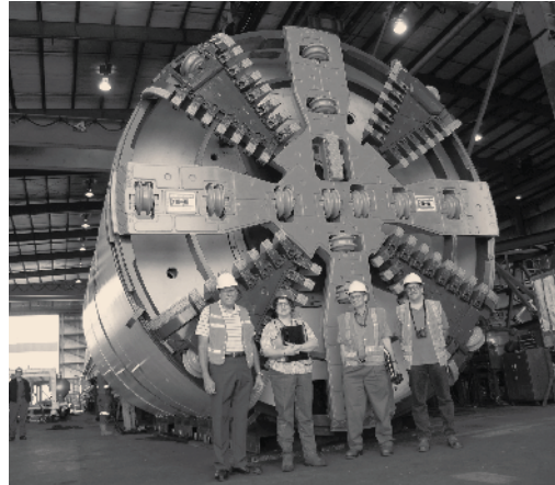
The Brightwater tunnel project used state-of-the-art boring machines to complete the underground work.
