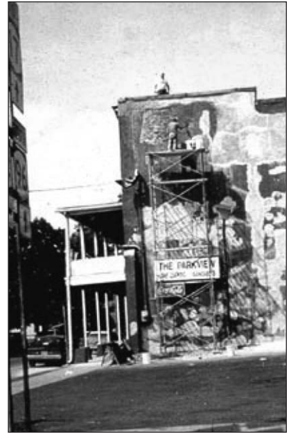
No fall protection here, either.
