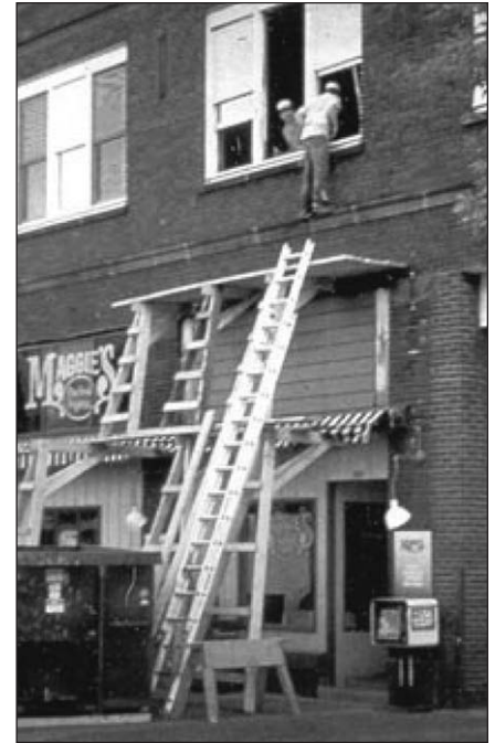
Out of the window, stepping on a ledge and over the second stage of an illegal scaffold...
