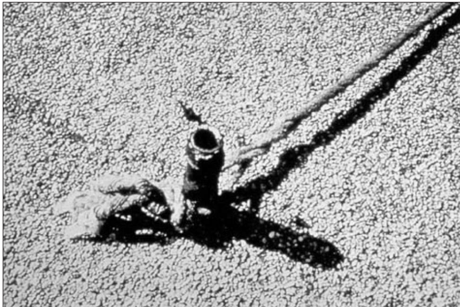
Let's hope that neither the pipe nor the rope is part of the anchor for a worker's lifeline. Neither one would meet the requirement of withstanding 5,000 lbs. of dead weight per worker tied to it...
