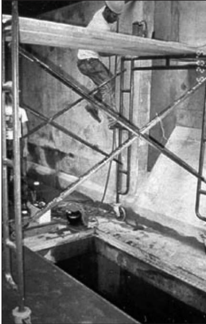
Worker is climbing a portable scaffold over an uncovered floor hole. No fall protection is being used, although total fall would be more than 10 feet above lower level.
