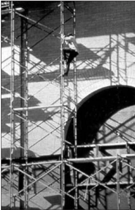
This worker is climbing the scaffold frame. He has no fall protection and unsafe access.
