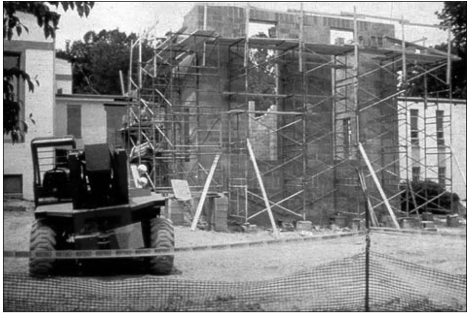
This is a different view of the same scene. Notice that the scaffold sections are sitting on blocks and propped up with planks. The entire scaffold could collapse if planks move or blocks shift.
