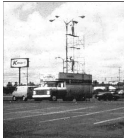
The roof of this truck is not a solid platform for the scaffold above it...
