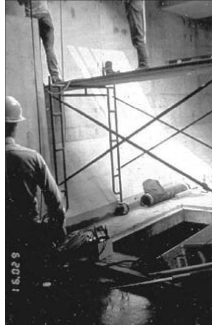
Different view of the same scene: the floor hole is not covered and workers have no fall protection.
