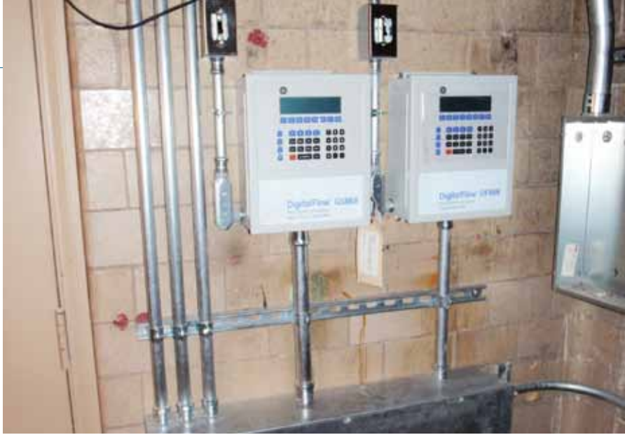
Tank monitoring systems were installed under the Capitol Complex Metering Program.
