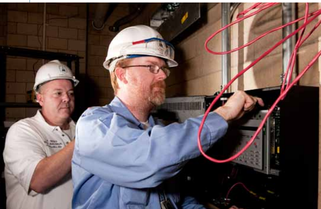
Electricians inspect equipment to ensure that critical systems are functioning properly.
