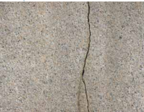
Although stone provides a solid long-lasting building material, cracks and fissures can weaken stone as it ages.
