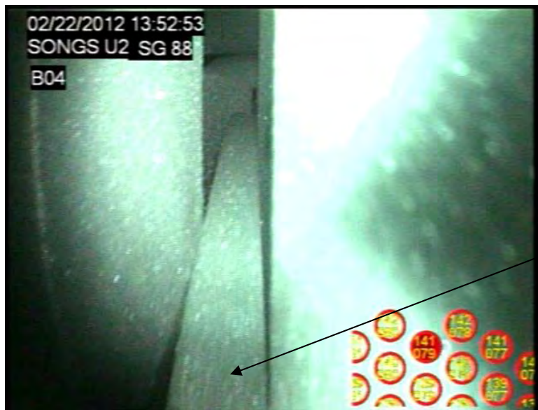
Photo-3 Visual Inspection Image of Outermost Tube Region [Unit-2B]
