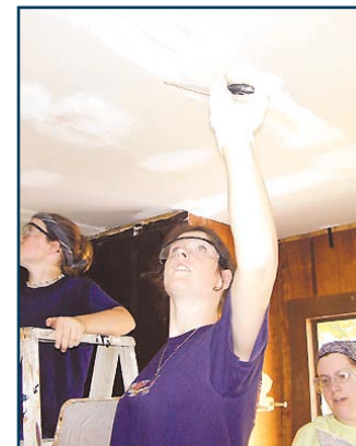
A TFHRC employee led a student volunteer group that helped to repair homes for families in southeastern Virginia during “Work Camp 2004.”
