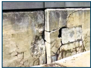
Concrete damage caused by alkali-silica reaction (ASR)
