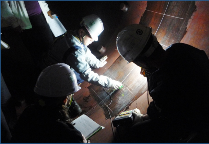
An NRC new reactor vendor inspector observes ultrasonic testing inside a steam generator.
