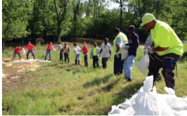
Workers place sandbags near a developing sand boil during the high water event of 2011.
