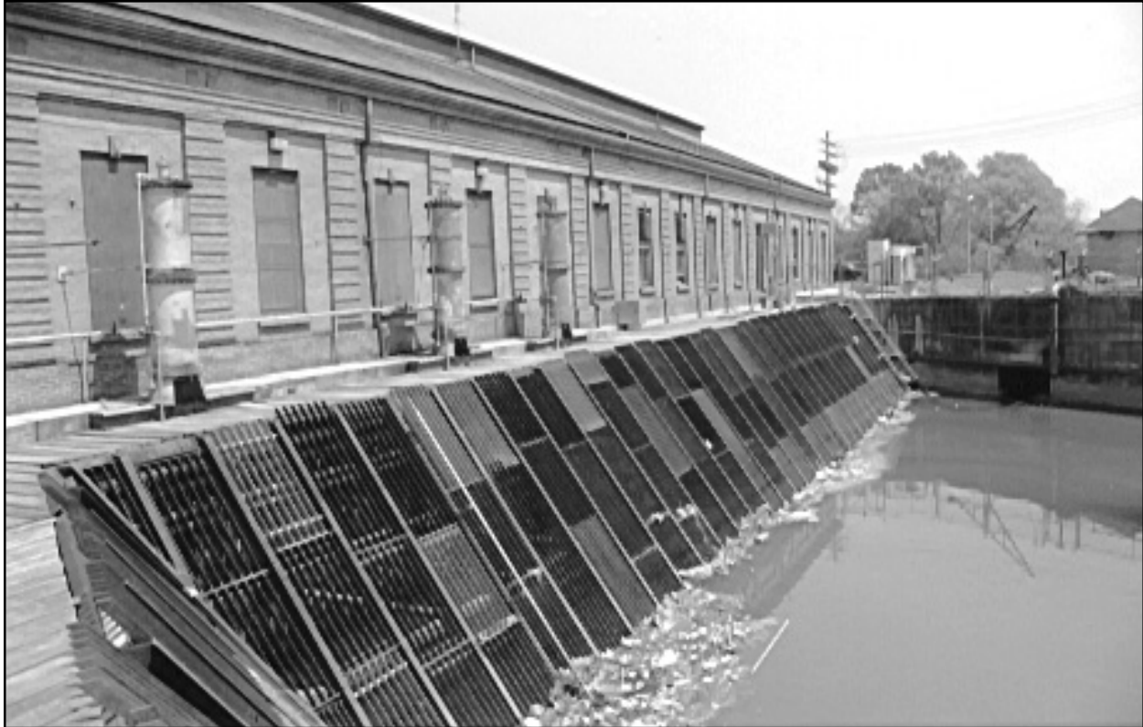
Figure 63. Drainage Pumping Station No. 7. Viewed from the northeast, showing trash screen and hydraulic sluice gate mechanisms.
