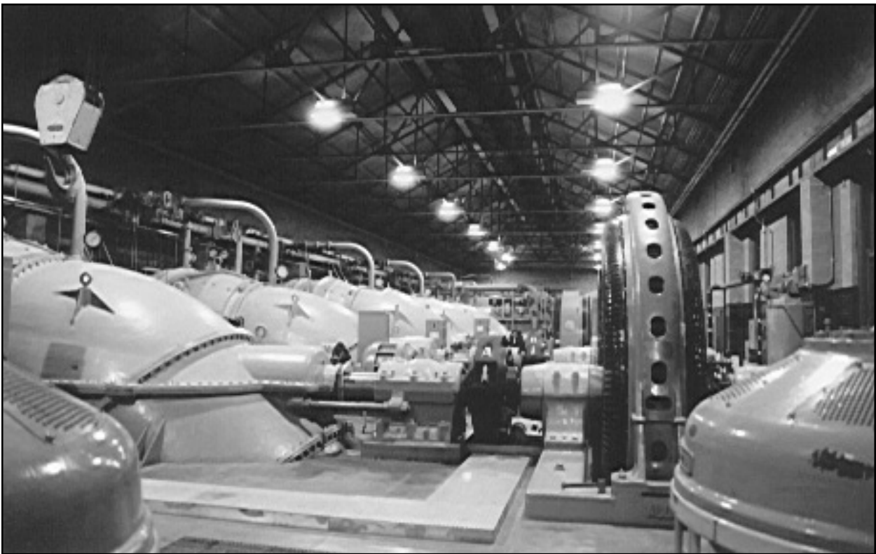
Figure 60. Drainage Pumping Station No. 6. View of interior looking east; in the foreground are 250 cfs vertical centrifugal pump motors. The remainder of the pumps are Wood screw pumps; in the foreground are two 12' pumps, and in the background are four 14' pumps.
