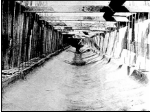
Figure 69. Interior of the Hagan Avenue Canal, shown during construction, ca. 1906. This concrete-lined and covered canal was constructed 1904-1906 (from Sewerage & Water Board 1906a).
