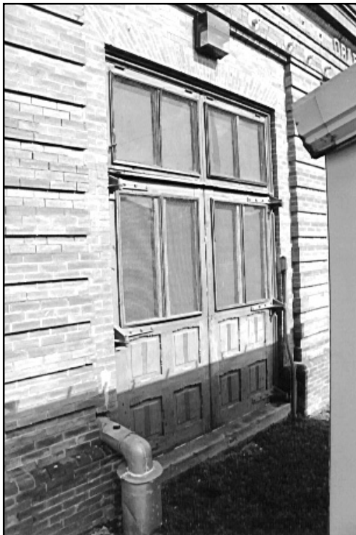
Figure 66. Drainage Pumping Station No. 7. Wooden vehicle door on west end of building.
