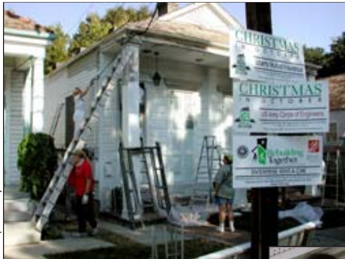
Left: Three different teams worked together to repair the house at 1728 Dante St.
