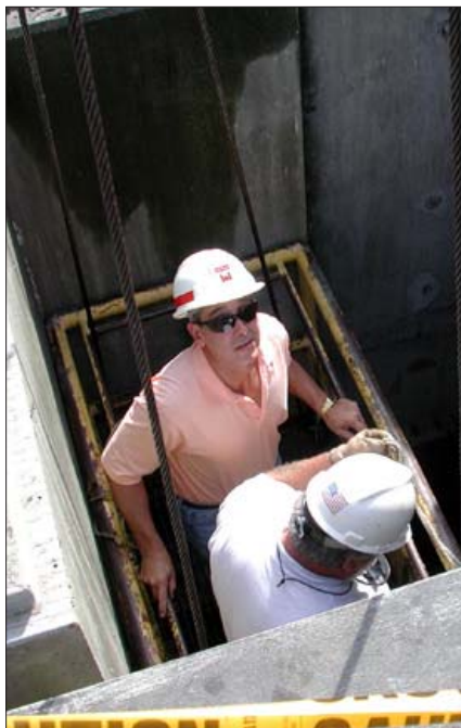
Chris Accardo, chief, Physical Support Branch, descends into a gate bay with Tim Hart, Operations, for an inspection.
