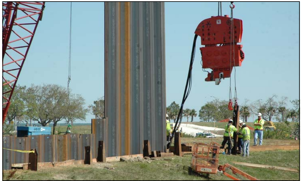
A significant number of construction contracts will be awarded in the next three to four months by the U.S. Army Corps of Engineers. The work will involve levee construction and repair, pump station renovation and repair, floodwall construction, and other hurricane protection work. (USACE Photo)
