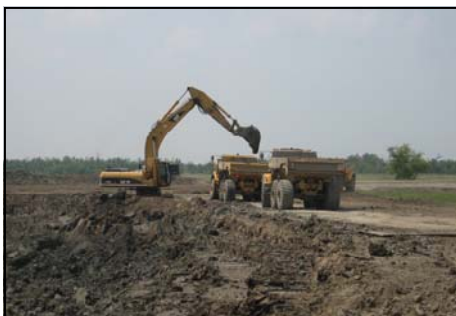
New construction contracts will involve collection and transportation of needed borrow material. (USACE Photo)
