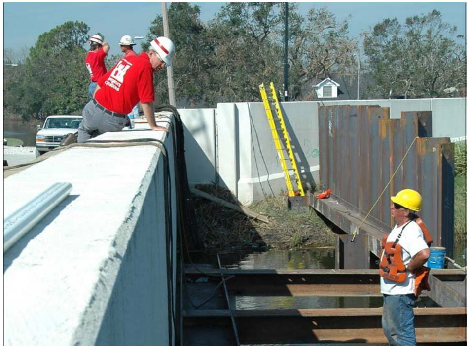
When complete, the WBV project will consist of approximately 70 miles of levees, floodwalls, floodgates and other water control structures for the West Bank area.
