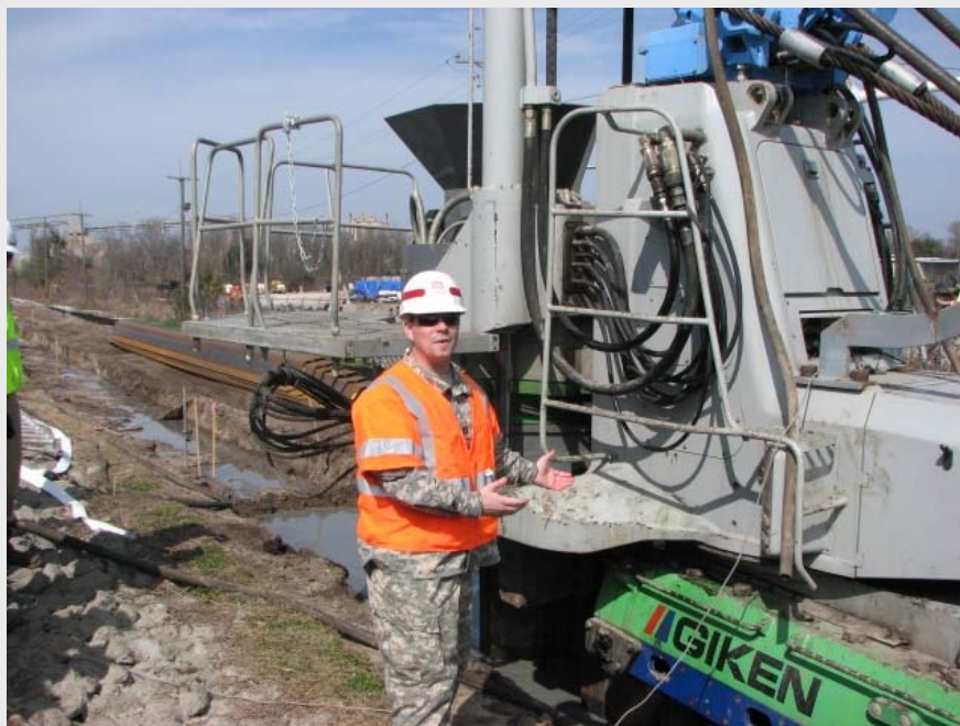
Capt. Nick Cali explains how the press-in method of pile driving works at the East Wall construction site.
