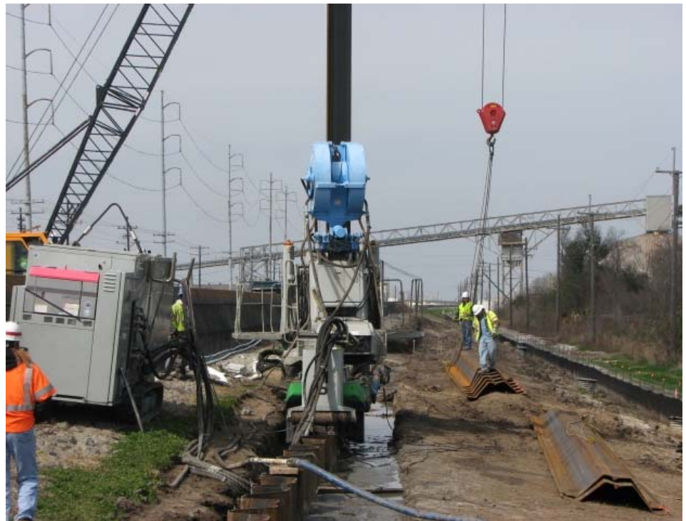
A silent piler is being used (above) along the East Wall on the Industrial Canal. The machine uses a hydraulic press-in method to drive sheet piles. This relatively new method is especially useful in constricted construction areas and in dense soils - like the conditions at the East Wall. USACE Photos
