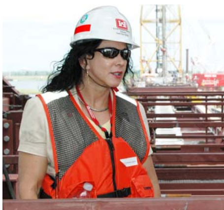
Karen Durham-Aguilera inspects work at the IHNC Surge Barrier on a recent visit.
