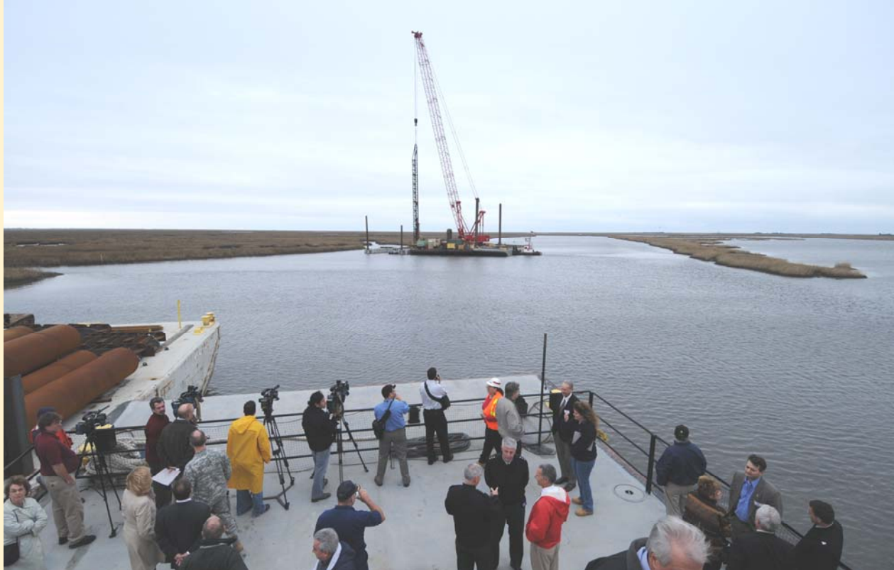
Corps personnel, VIPs and the members of the press gather on the bow of a Corps barge to view pile driving activities for the monumental IHNC Surge Barrier project.
