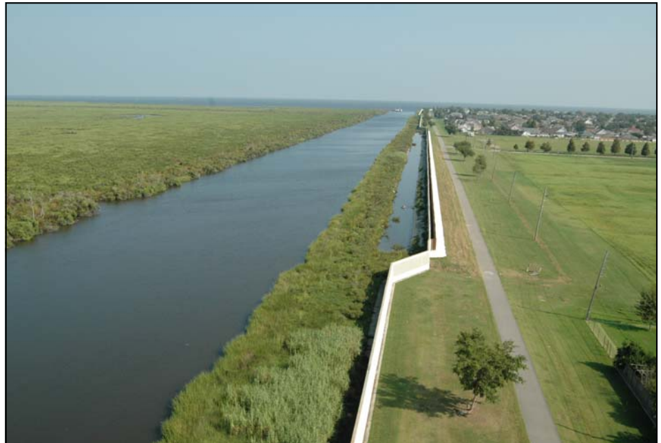
This section of floodwall is part of the repair work done to the Lake Pontchartrain & Vicinity Hurricane Protection Project. The Corps of Engineers repaired 220 miles of levees and floodwalls from September 1, 2005 to June 1, 2006, the start of the 2006 Hurricane Season. (USACE Photo)
