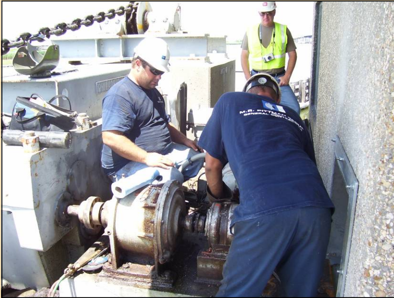
From left, Jeff Binder and Jeffery Pelegrin, both with M.R. Pittman Group, work on the motor for the Empire Flood Gate in Empire, LA. Standing in the background is Corps of Engineers Project Manager Larry Wernle. (USACE Photo by Bob Lord)
