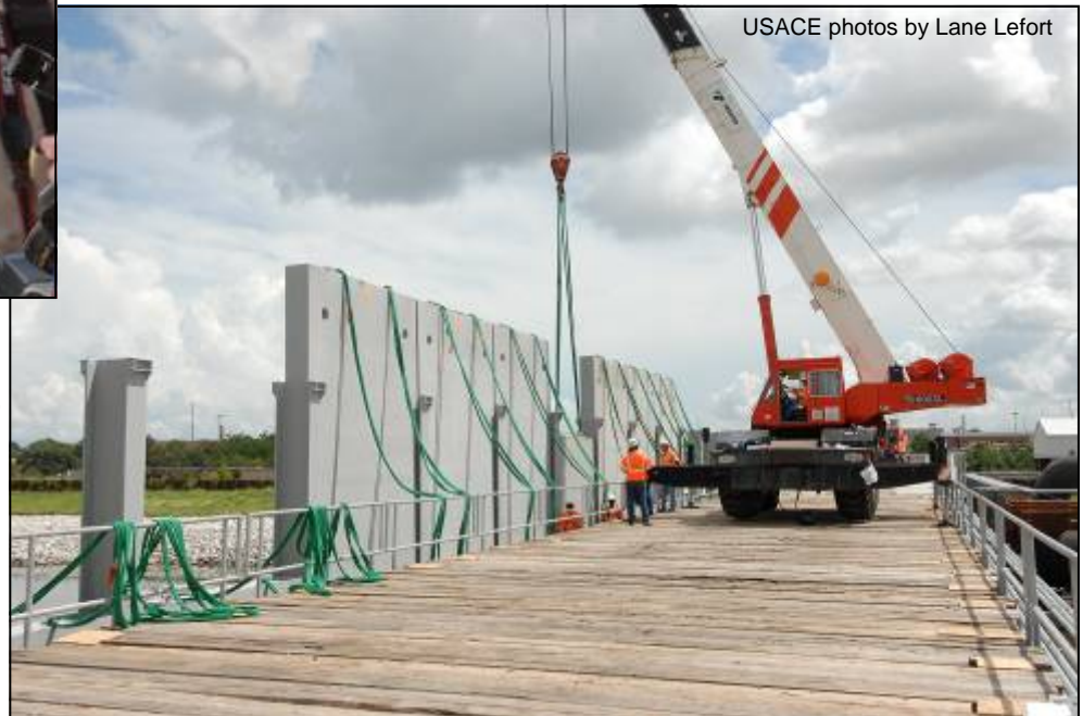
Corps technicians use a crane to lower one of the closure gates at the London Ave. Canal demonstration. Lowering nine of the 11-gate system took less than 10 minutes, as each gate smoothly slipped into its place.
