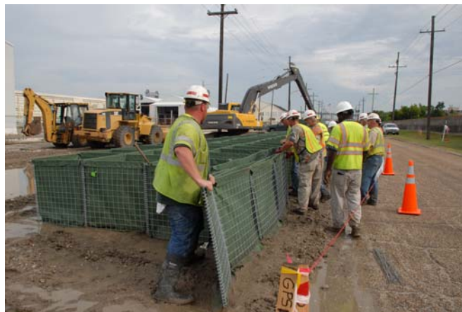
Workmen unload and assemble HESCO baskets to be placed at the IHNC.
