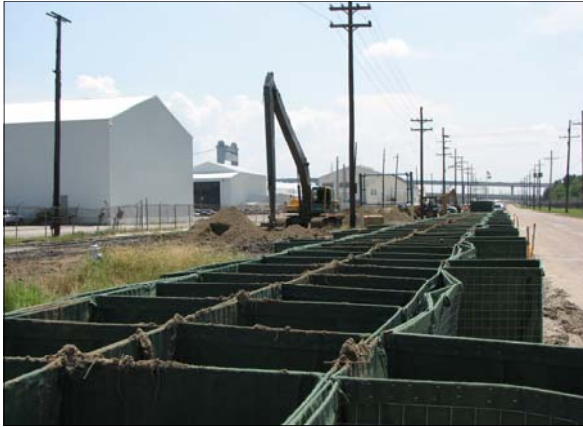
Assembled HESCO baskets to be used at the IHNC are filled with sand.
