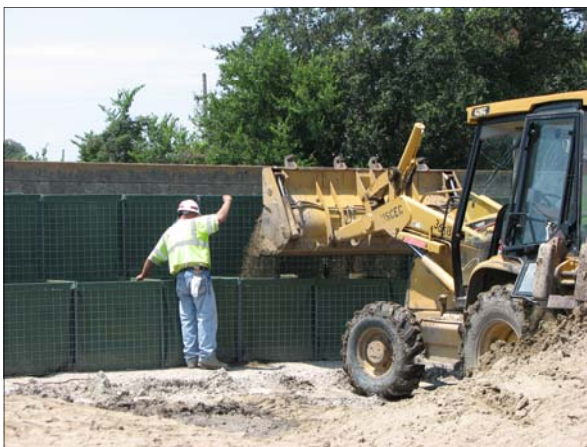
Workers place HESCO baskets at the IHNC floodwall. The Corps will con-
