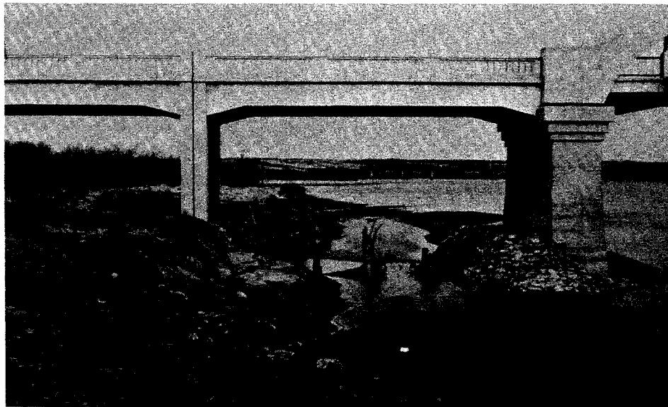
Figure 246. Erosion of left bank at PH-5 bridge, November 7, 1960.
