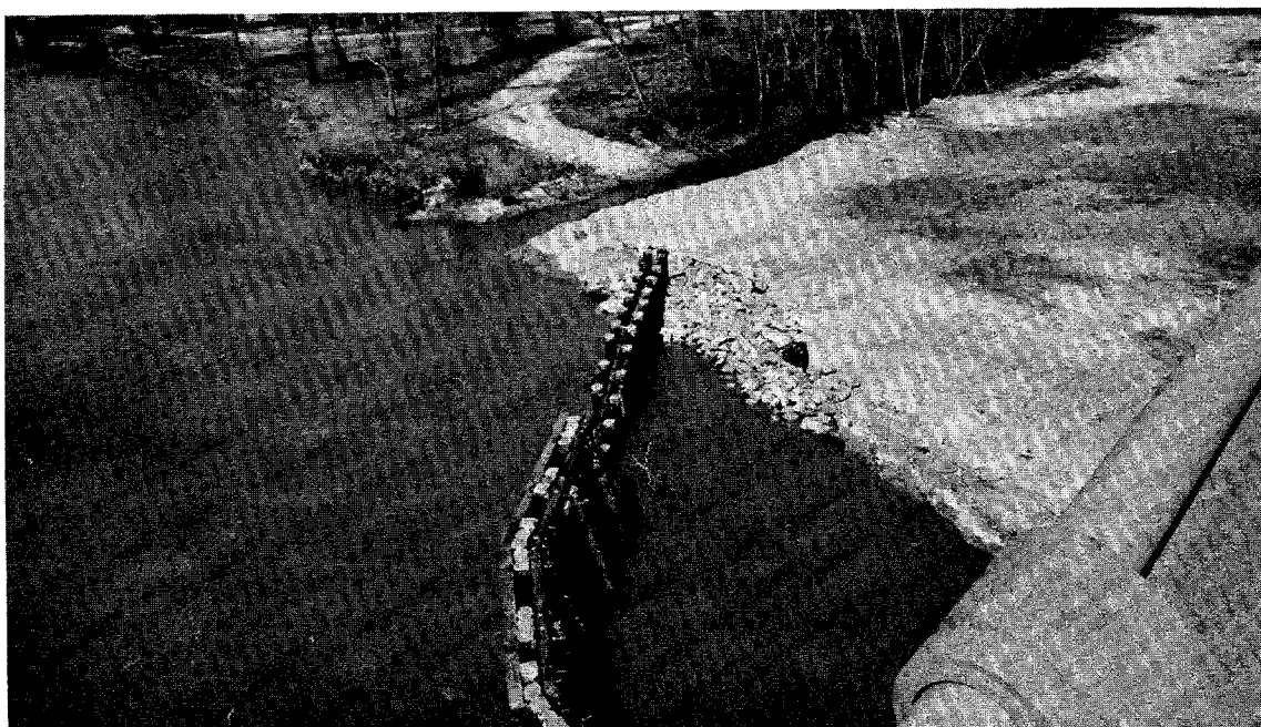
Figure 91. View on March 2, 1977 of upstream end of left timber-pile fender as extended to bank by addition of a double row of timber piles.
