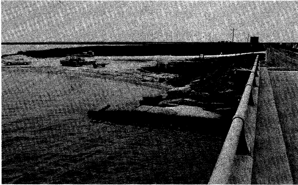
Figure 120. View of upstream side of left bridge abutment, Sabine Pass at SR-82, on March 9, 1977, showing erosion behind concrete blocks.
