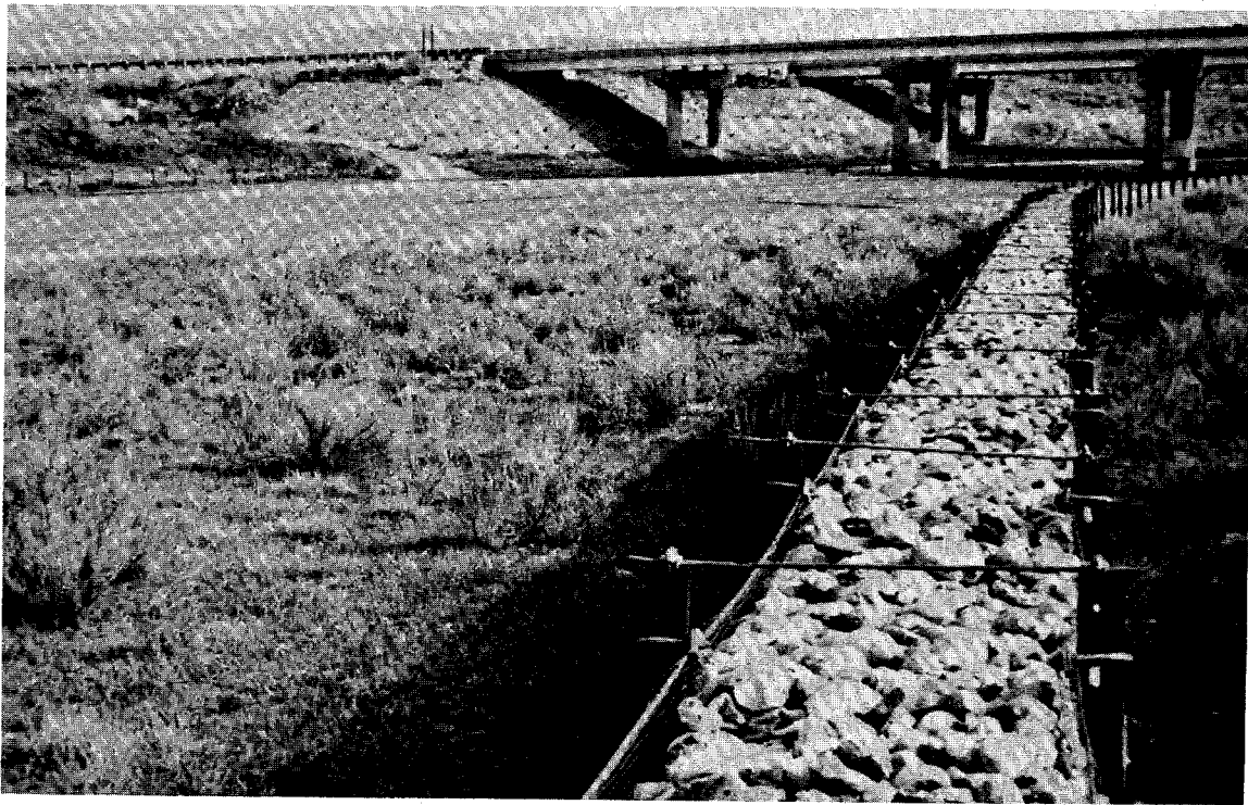
Figure 290. View looking downstream along spur dike (training dike) at I-25 bridge, in April, 1977. Rock-and-wire mattress on abutment fill-slopes is visible in background.
