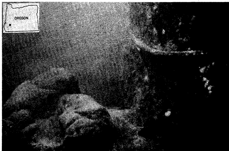
Figure 298. Underwater view of cylindrical pier showing exposed reinforcing steel. Abrasion damage extends to the streambed of cobbles and boulders. (From Oregon Dept. of Highways.)
