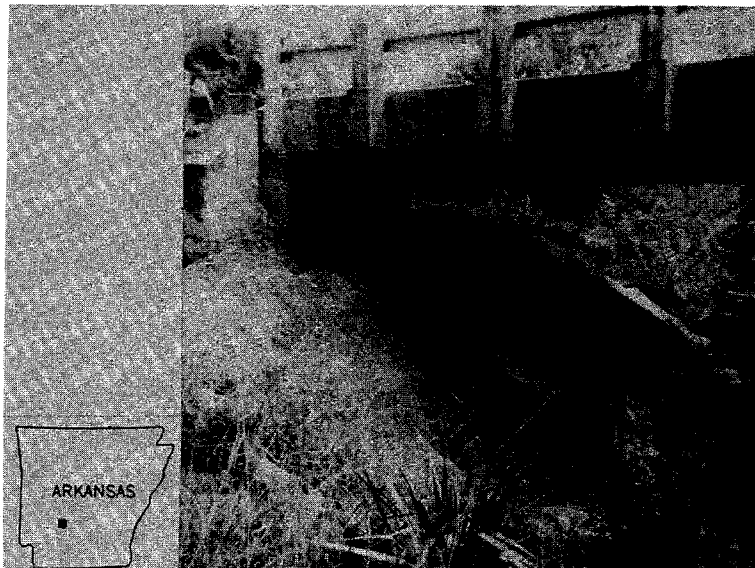
Figure 36. View of failed concrete pavement at left abutment of SR-9 bridge, April 28, 1976.
