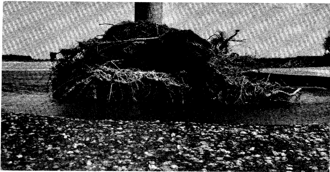
Figure 7. Debris lodged on exposed pier footings. (From Calif. Dept. of Transportation, photograph taken prior to 1976.)
