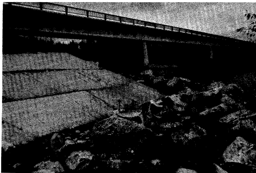
Figure 7. View of riprap launching apron, upstream side of left abutment of PH-587 bridge, on September 29, 1977.
