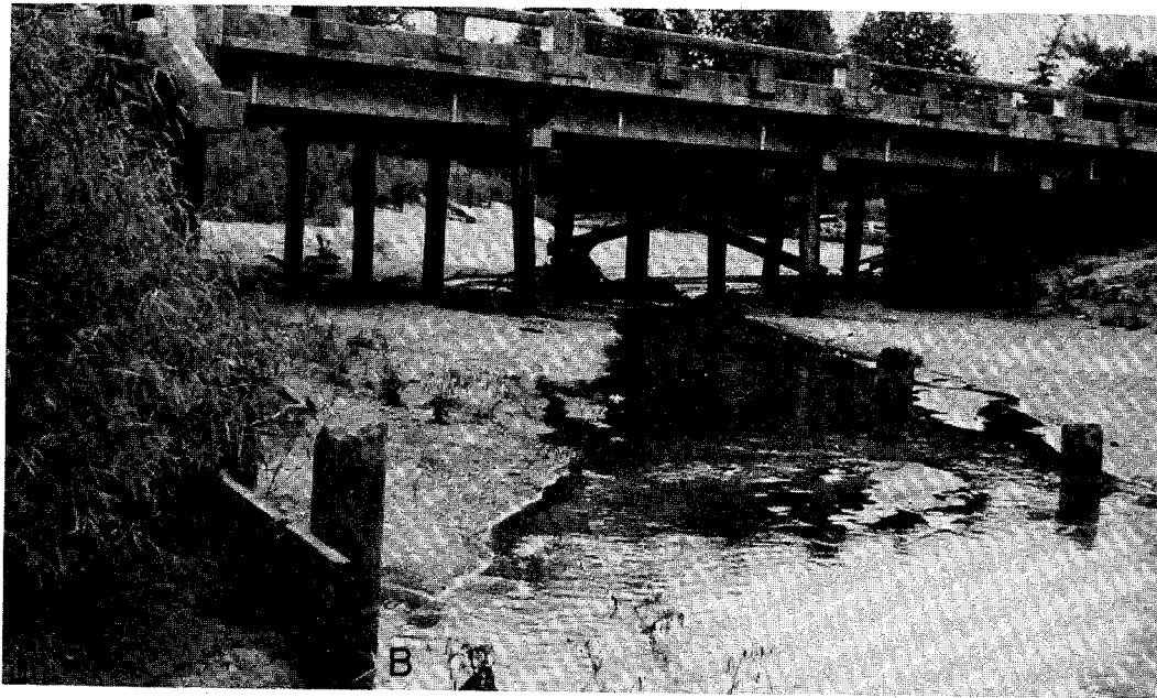
Figure 177. A, upstream view from bridge of timber-pile bulkhead and car-body revetment along left bank of Hooker Hollow Creek, on June 1, 1976. B, upstream view toward bridge showing bank recession at right abutment (left side of photo).
