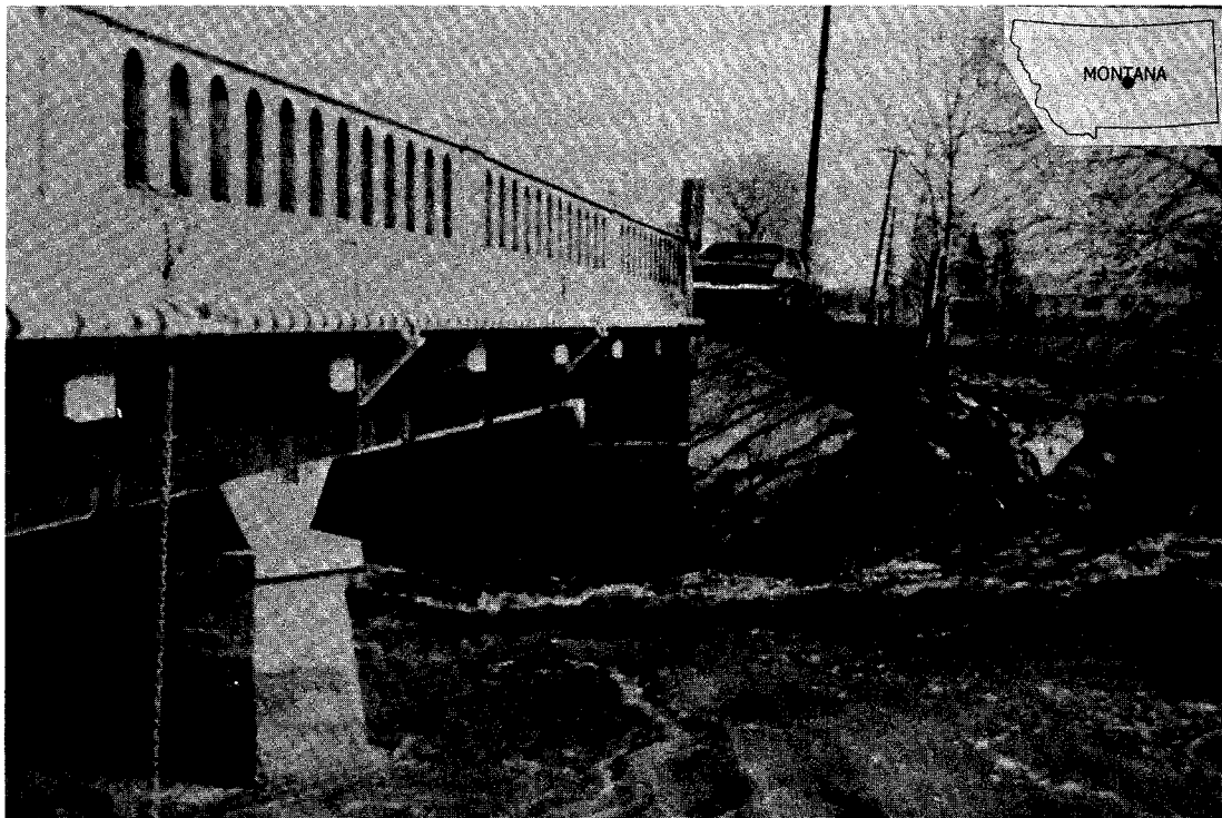
Figure 203. View of right abutment of US-191 bridge in May, 1975, after undermining and subsidence of abutment footing. (From Montana Dept. of Highways.)
