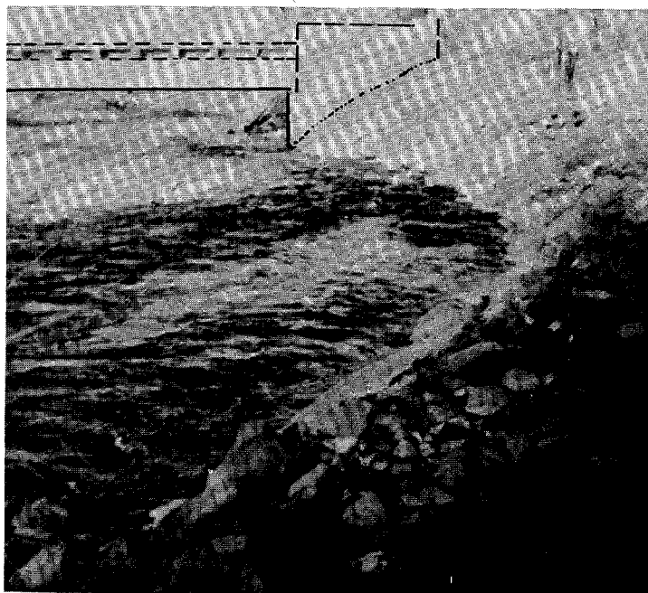
Figure 202. Downstream view of riprapped bank and right abutment, I-25 bridge at Boulder River. (From Montana Dept. of Highways.)
