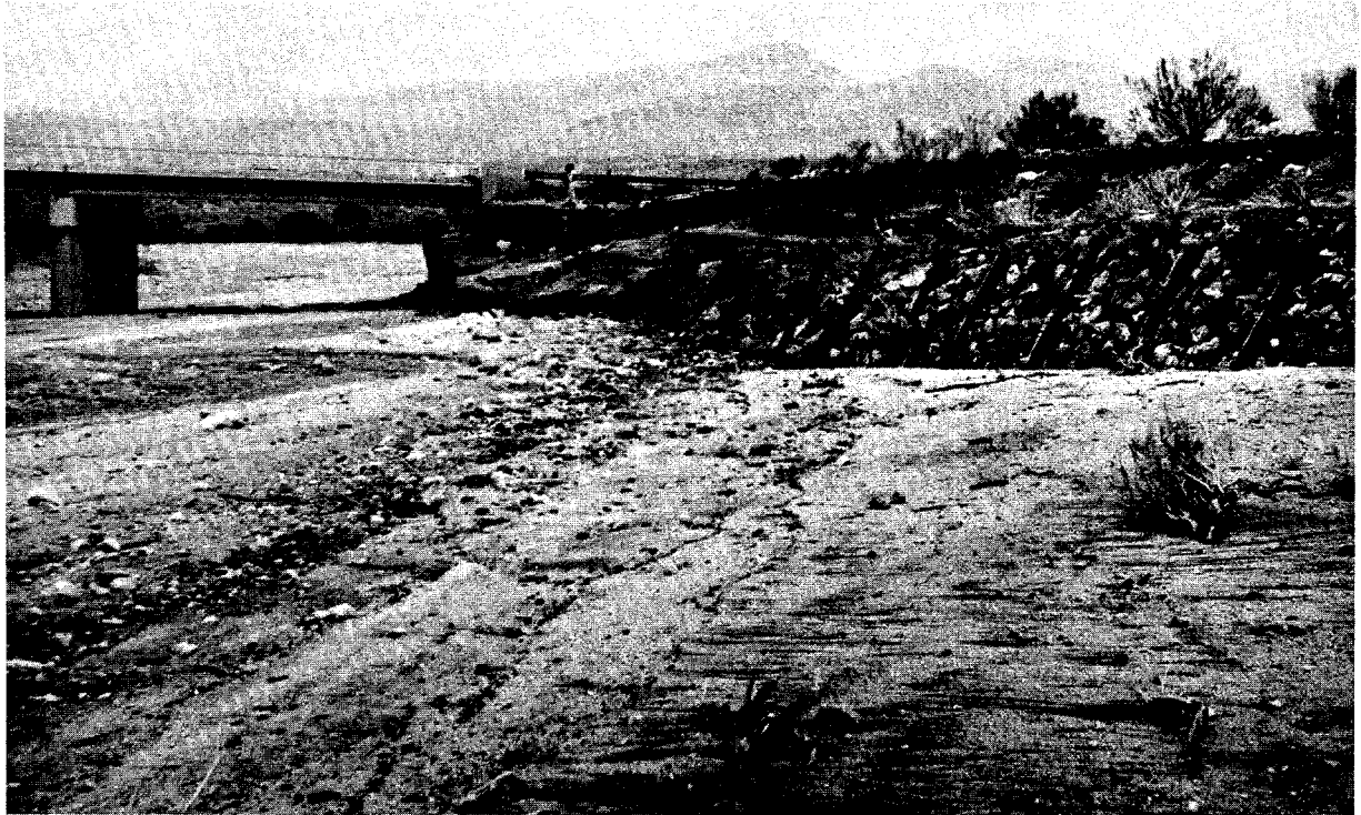
Figure 209. Damaged railbank protection on right bank upstream from bridge after August 1971 flood. (From Arizona Dept. of Highways.)
