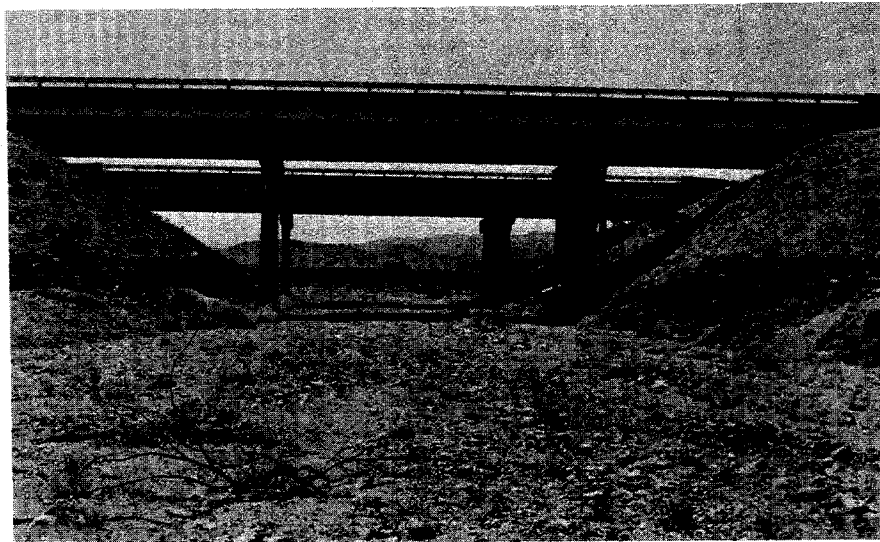
Figure 68. View upstream in 1976 of wire-enclosed riprap as repaired after the 1972 flood.
