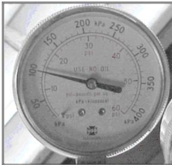
Figure D-5 - Gauge Measuring Hydrogen Line Pressure
