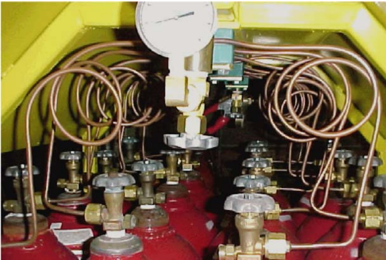
Figure K-6 - Unauthorized Manifolding of Cylinders
