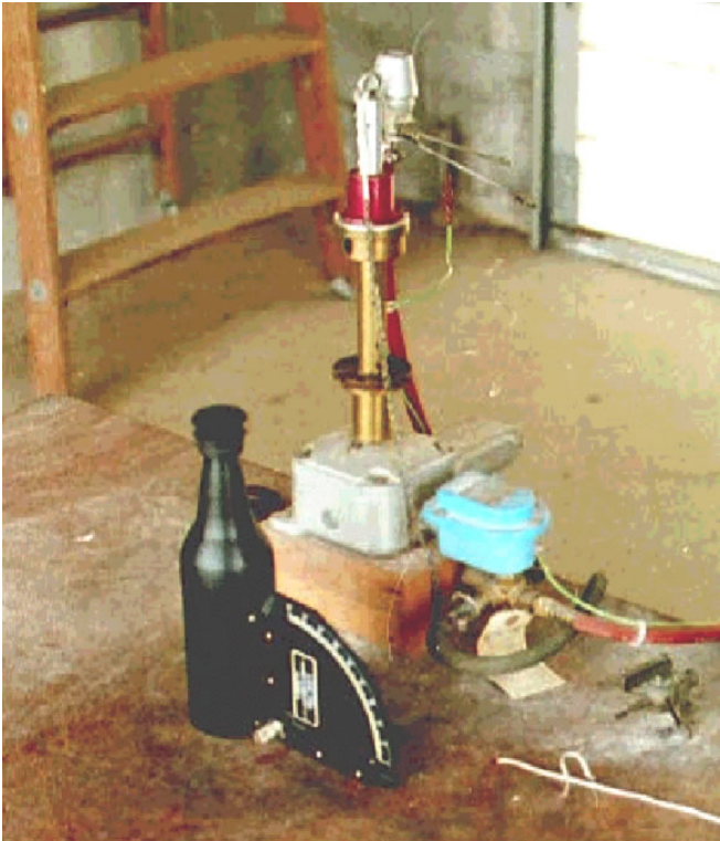
K-5 - Unauthorized Hose
