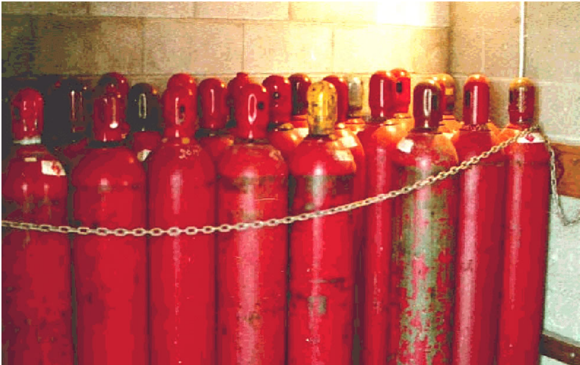
Figure K-1 - Cylinders Secured Improperly
