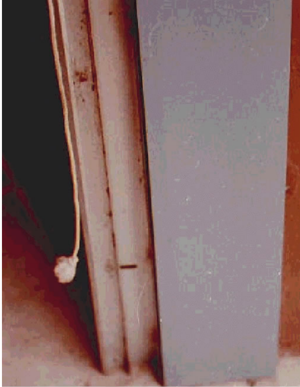
Figure K-3 - Ungrounded Overhead Door Railing
