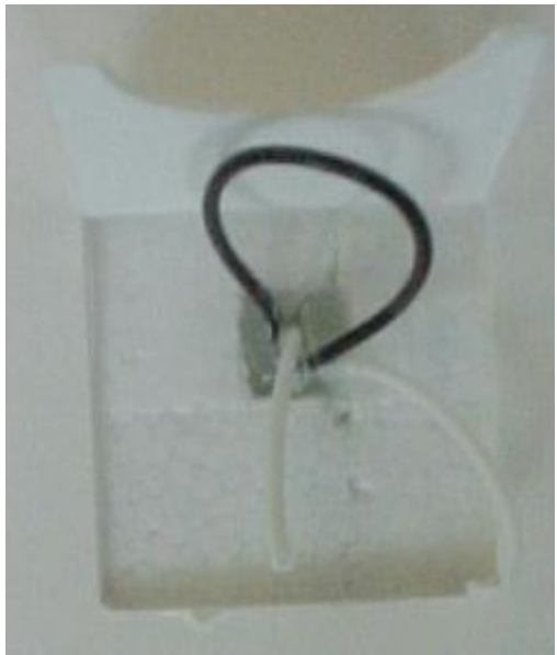
Figure N-9 – Cut Wires
