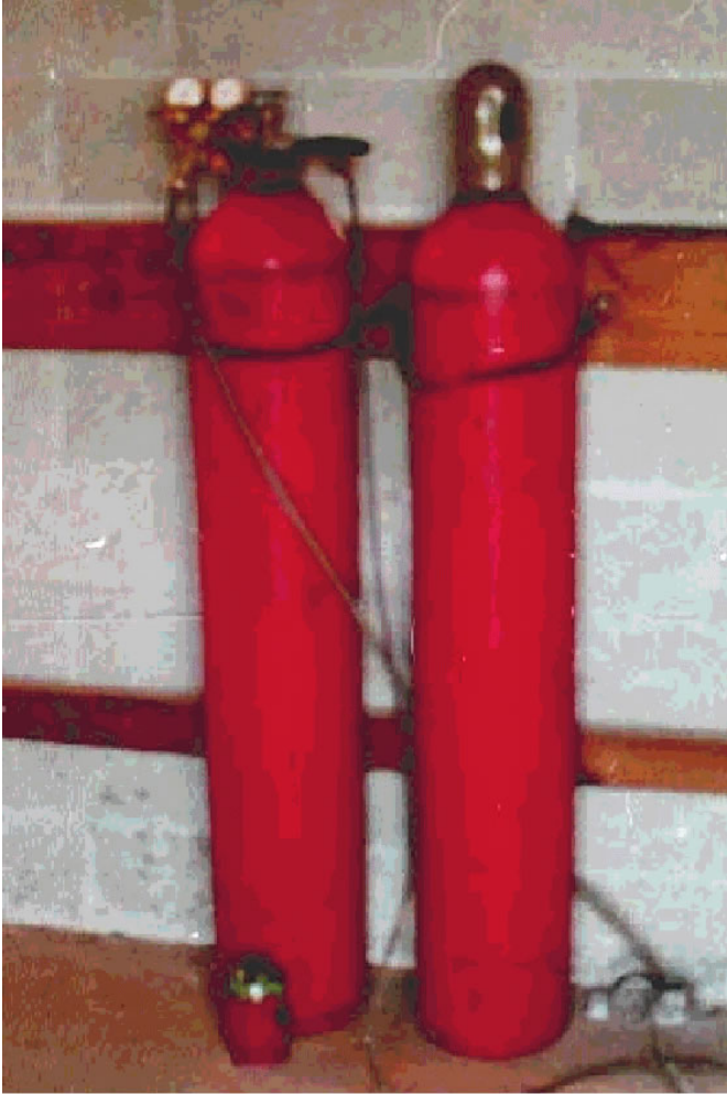
Figure K-2 - Properly Secured Cylinders
