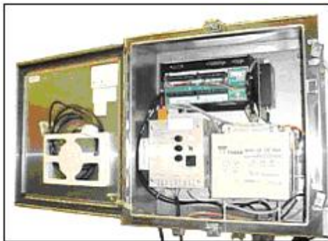
Figure L-7 – Remote Processing Unit (RPU)
