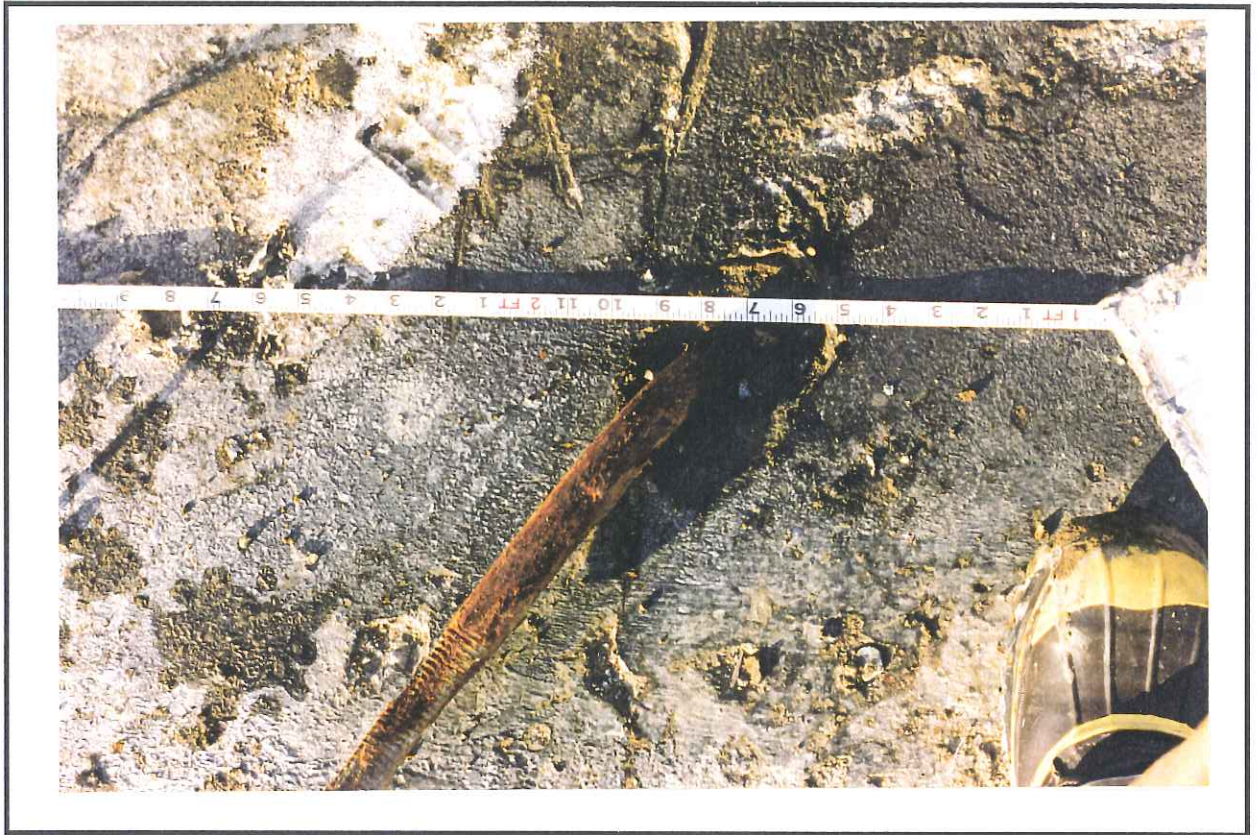
Photo 8 - 10 AN Scrubber Mounting Bolts
