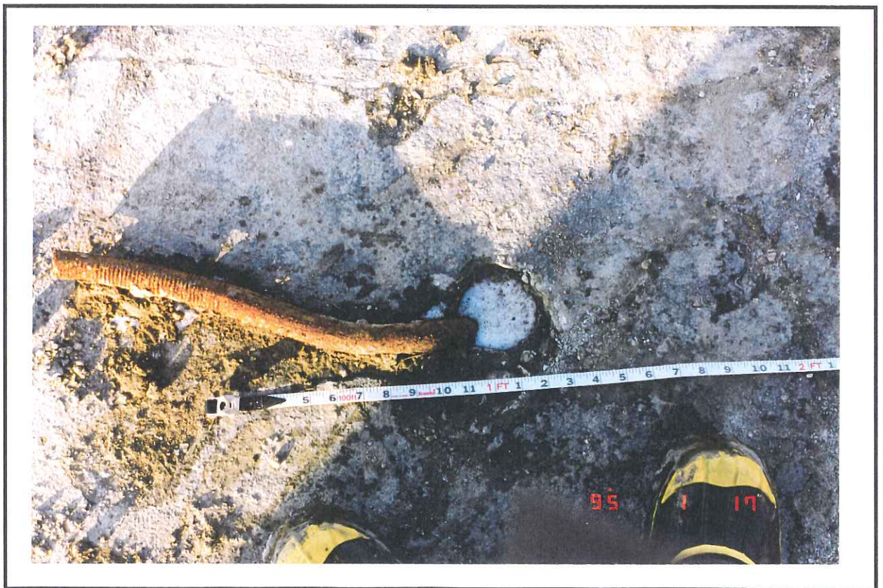
Photo 8 - 11 AN Scrubber Mounting Bolts
