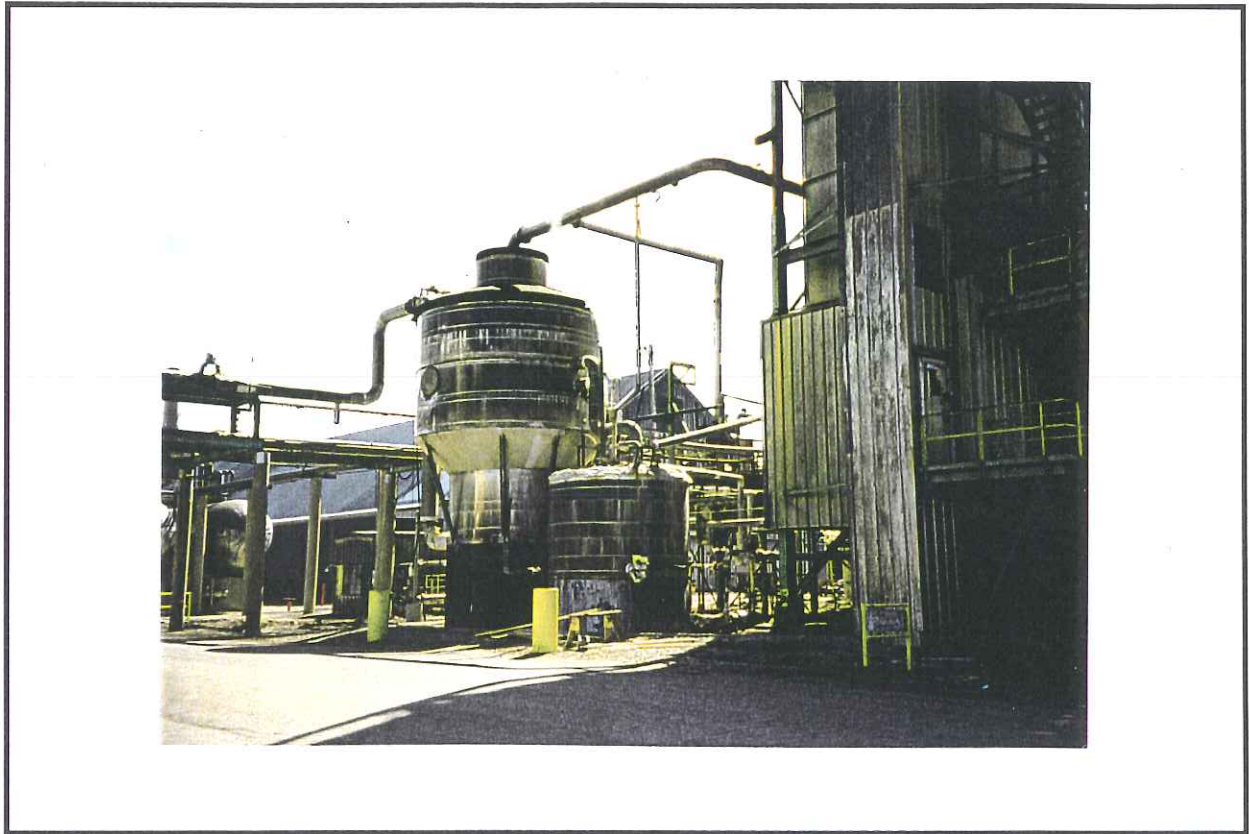
Photo 5 - 1 Neutralizer and Rundown Tank
