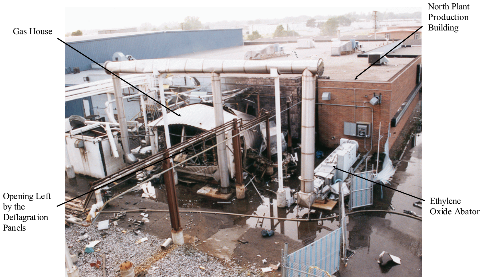
A-1: The Gas House and the Production Building after the explosion and fire.
