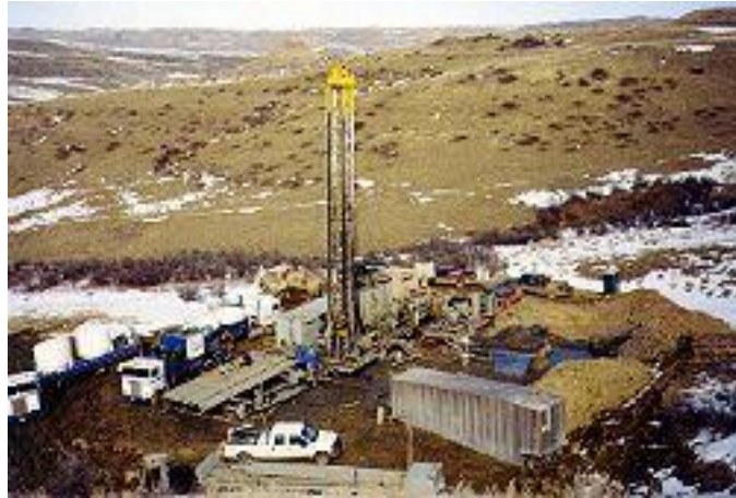
Figure 8 - Photo of Coal Bed Methane Well.
