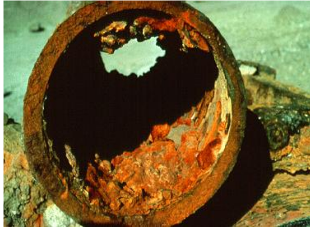
Salinity damages to municipal water pipe.
