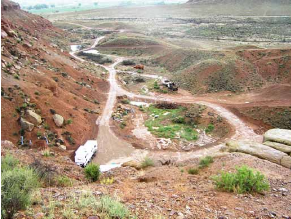
Figure 29. June 1, 2009, rainstorm tests the newly built “gully plugs” on south end of property
