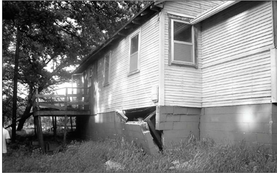
Figure 2-8. The walls of this basement in Iowa failed because of the pressure exerted by water and saturated soil.
