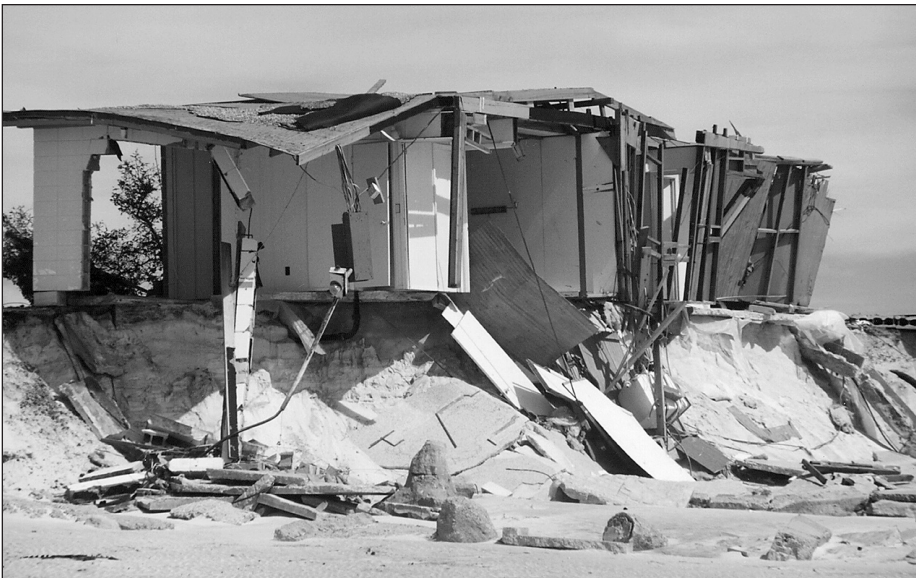
Figure 2-5. The extreme impact of large, fast-moving waves, combined with the removal of supporting soil by erosion and scour, can have devastating effects on buildings exposed to coastal flooding. This home along the Gulf of Mexico shoreline was destroyed during Hurricane Opal.
