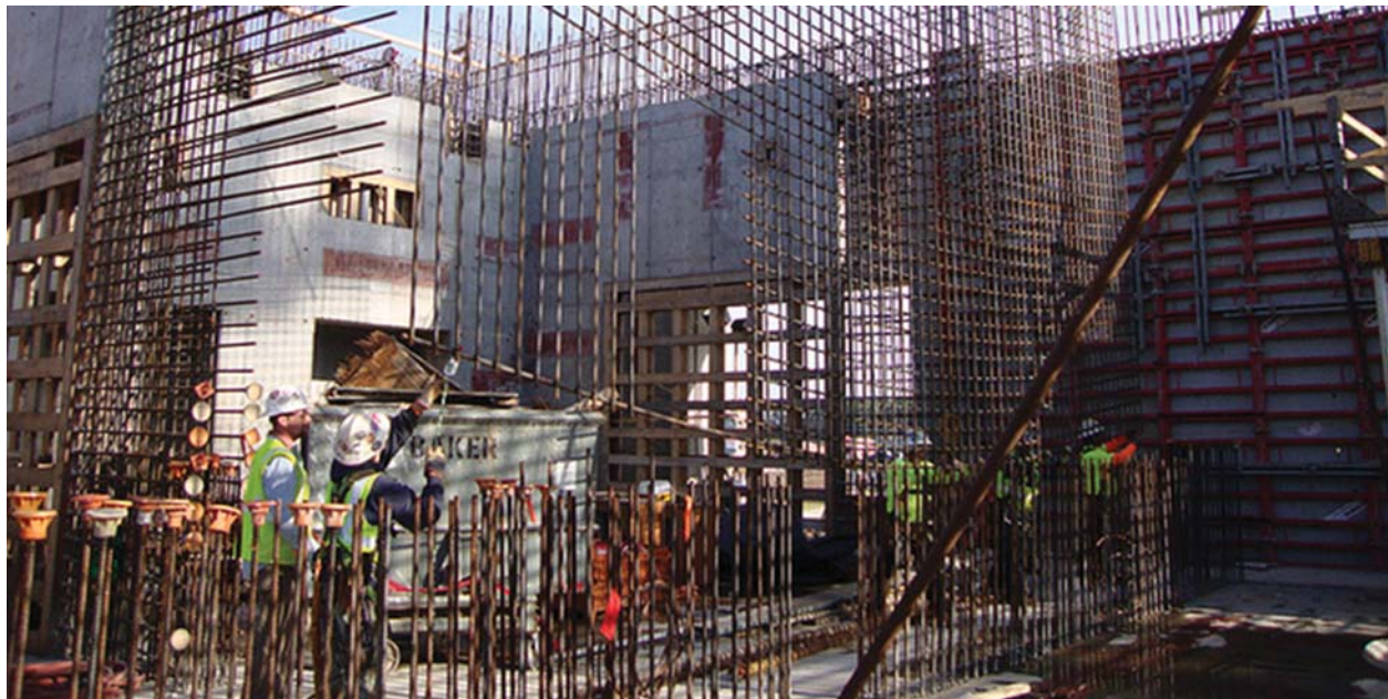
Installation of a rebar curtain at the Mixed Oxide (MOX) Fuel Fabrication Facility.
