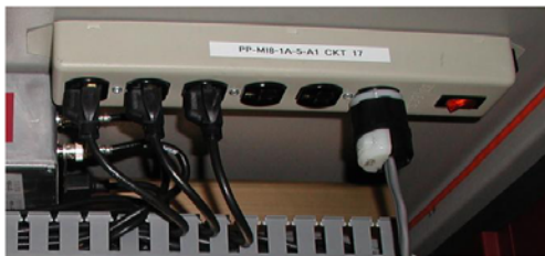
Figure 18. AC utility strip in "C" quadrant
