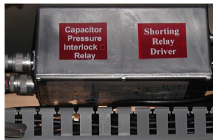
Figure 4. Interlock relay box in C quadrant.
