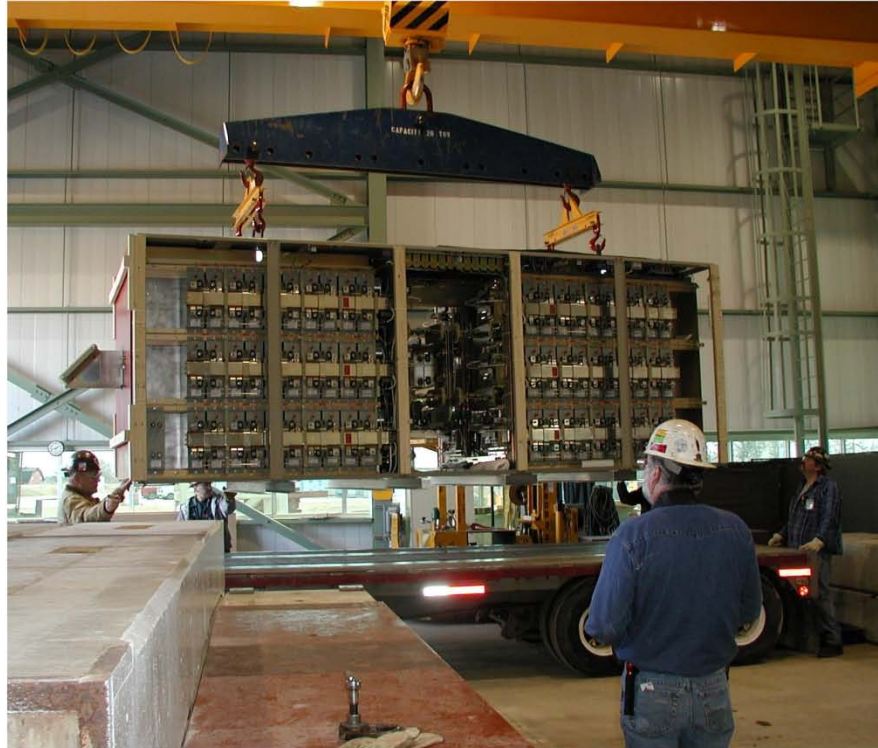
Figure 43. Spreader bar arrangement used for lifting or moving capacitor bank. Weight without doors installed is 22,000 lbs.
