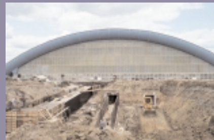
Construction of the beam line to the Meson Laboratory, where some of the first Tevatron fixed-target experiments took place in Fall of 1983.
