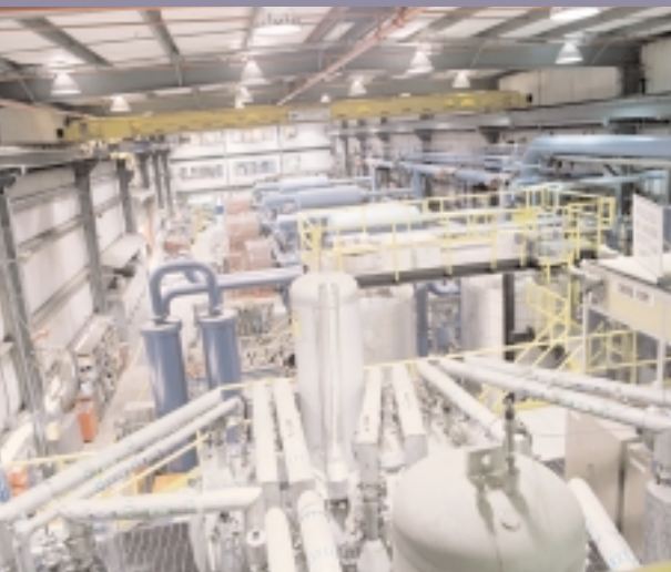
Fermilab's Central Helium Liquefier (CHL)
