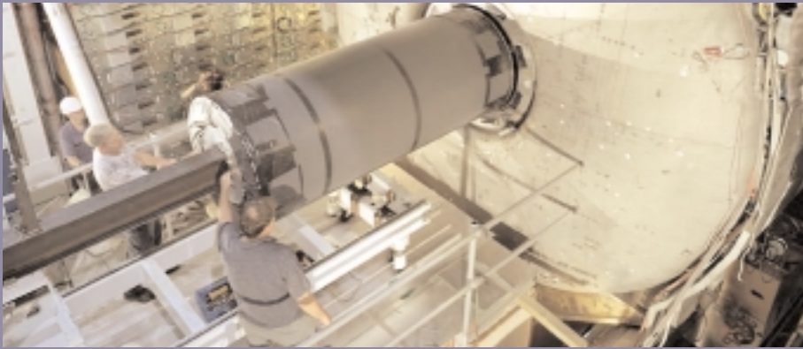
Central Fiber Tracker installation at DZero. Final placement of tracker into calorimeter.
