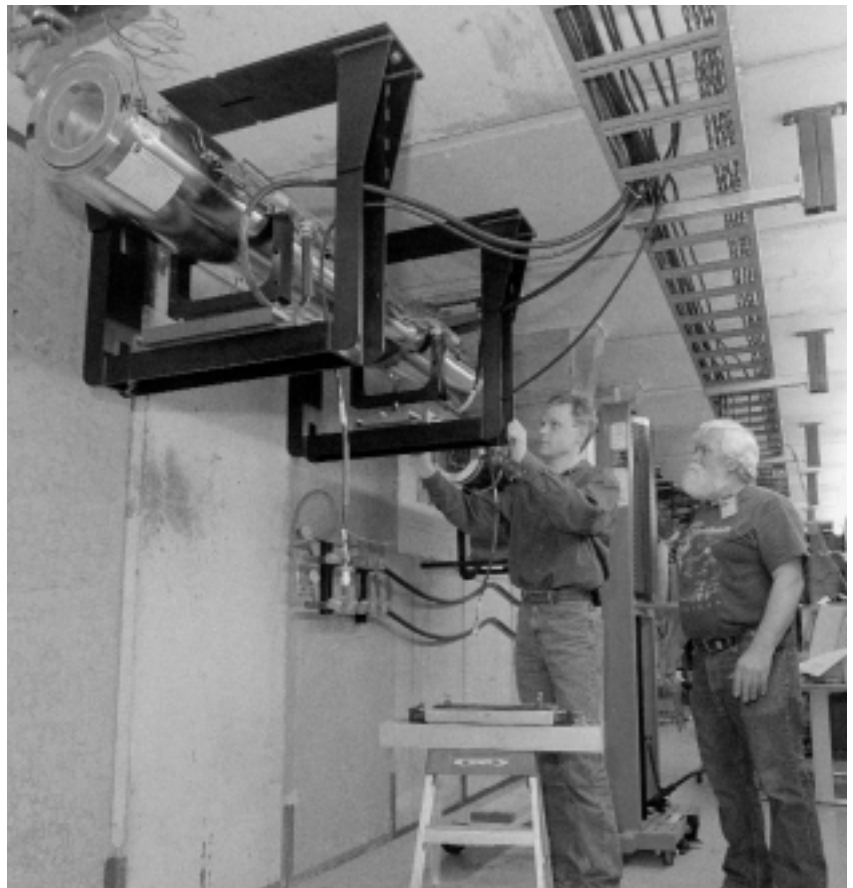
Project engineer Jerry Leibfritz (left) and Jerry Nelson install a 7-foot-long module of the cooling section, in which electrons will travel side by side with antiprotons.
