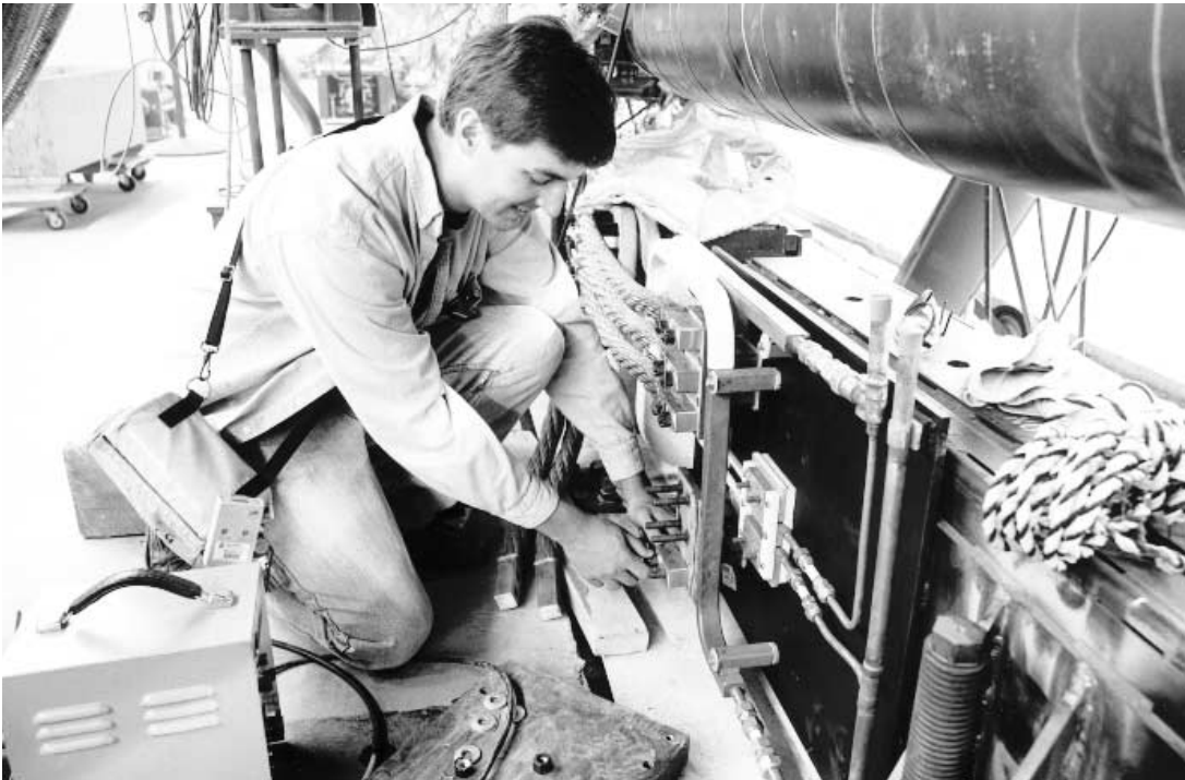
Operator Denton Morris connects electrical power source to Lambertson magnet that extracts proton beam from the Tevatron.
