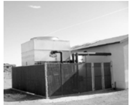
Fort Irwin, near Barstow, CA., is saving more than $169,000 each year in energy and water costs by using technologies such as this new cooling tower/heat exchanger system.
