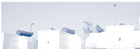
Fuel oil generators used for peak load shedding at the CDC Roybal Campus in Atlanta, Georgia.
