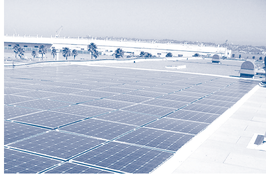
A 21.6 kilowatt photovoltaic system on Bldg 678, Naval Air Base Coronado, California.
