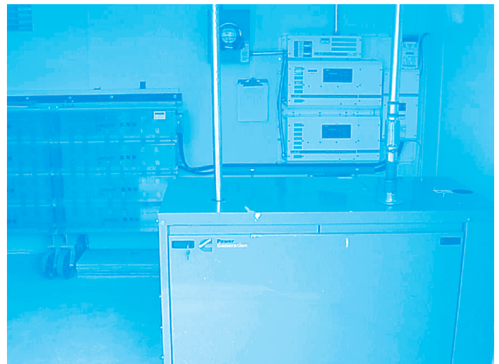
Hybrid power system consisting of propane-fueled generator, battery bank, and inverters inside generation/distribution building.
