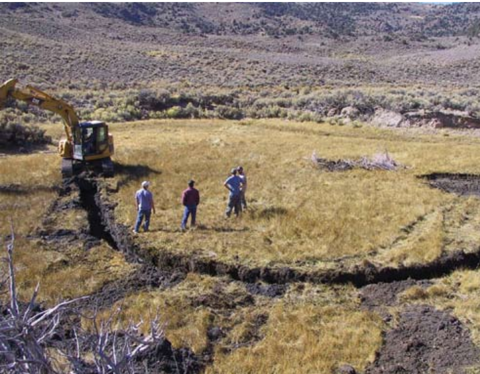
Upper photo: Construction of Horseshoe Pond begins. Lower photo: Horseshoe Pond after completion.
