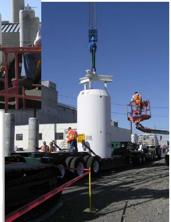
Interim Storage Container in position on the transporter
