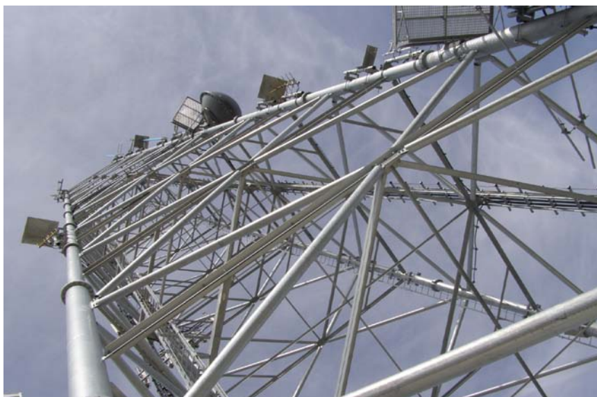
Tower and Antenna Arrays at CCCF
