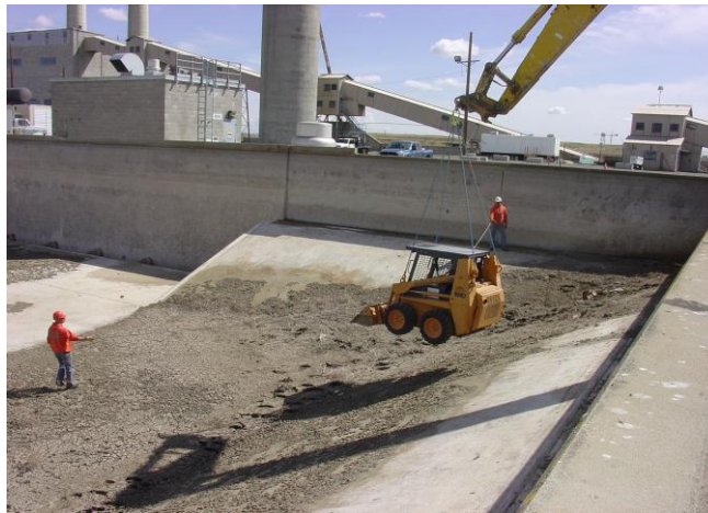
Refurbish 200E Raw Water Reservoir Project (Cleanup prior to Installation of Liner)
