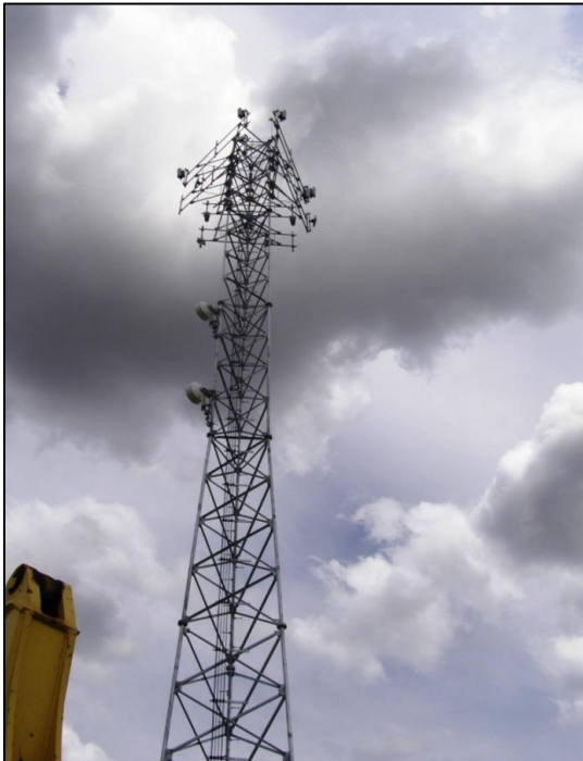
200East Communications Tower
