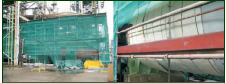
Field demonstration activities: installation of aerogels onto a variety of in-service hydrocarbon-processing equipment
