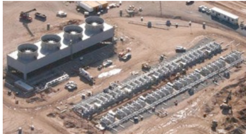
Figure 14. Raser's Hatch Power Plant in Beaver Creek, Utah
