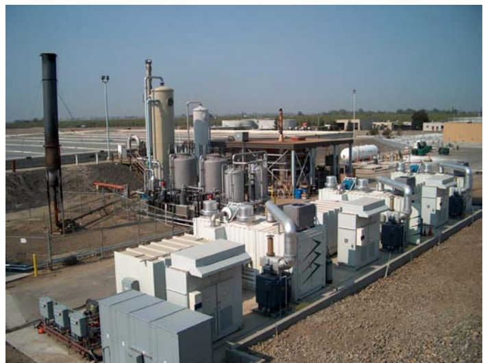
Figure 16: FuelCell Energy facility at the Tulare, California Wastewater Treatment Plant. Photo courtesy of FuelCell Energy, Inc., NREL/PIX 19193
