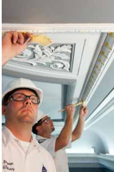
Above: Timothy Steadman and Charles Taylor, AOC Senate painters, carefully apply gold leafing within a Senate Committee room.
