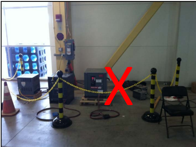
Electrical Hazard Areas
