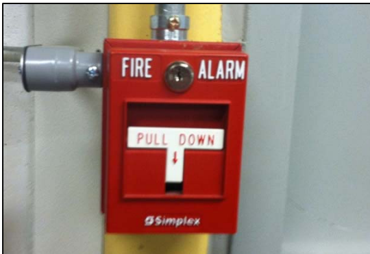
Fire Alarm Pull Box
