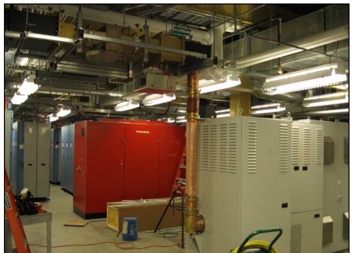
Figure 2. Booster RF transmitter installation in the Injector service bldg.
