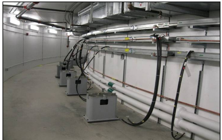
Figure 1. Booster arcs with complete cable trays, cables, DI-water piping and pedestals for magnet girders.
