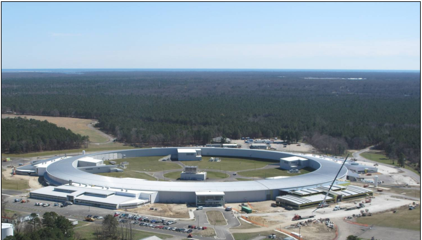
A crane moves the final bundle of metal roofing panels from a flatbed to the roof of pentant 5, late on the last workday in March.
