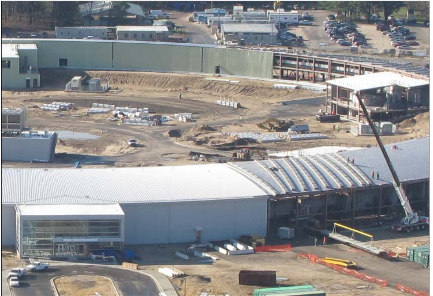
Early on the last workday in April, materials are being staged for the last section (pentant 5) of the standing seam metal roof.
