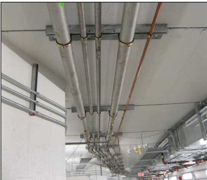
Figure 6. Water piping in the tunnel.
