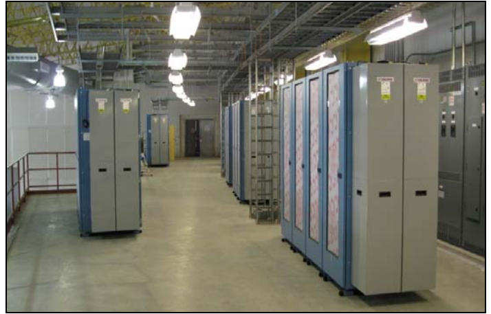
Figure 7. Equipment racks installed on the mezzanine.
