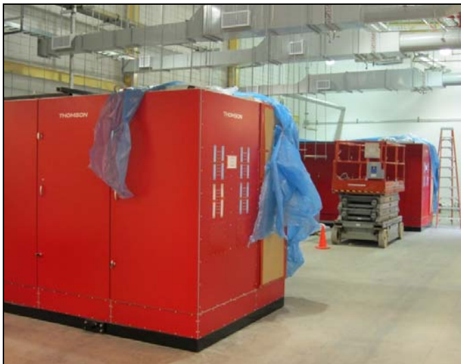
Figure 4. Delivered RF transmitter systems in the NSLS-II RF building.
